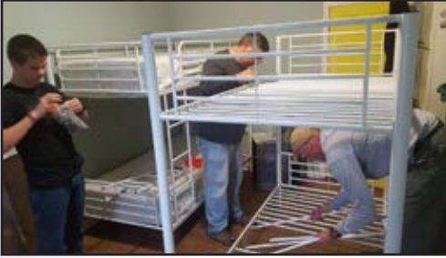
UM men of two North Carolina churches install new beds at Amy's House.
