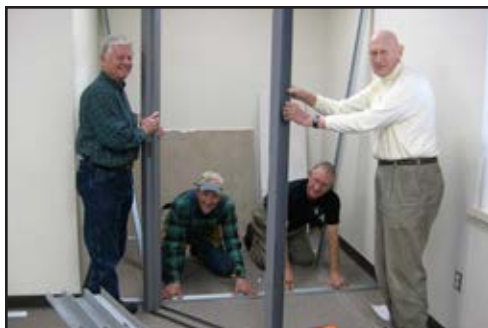
UM Men work on a classroom expansion at First UMC of Colleyville.
