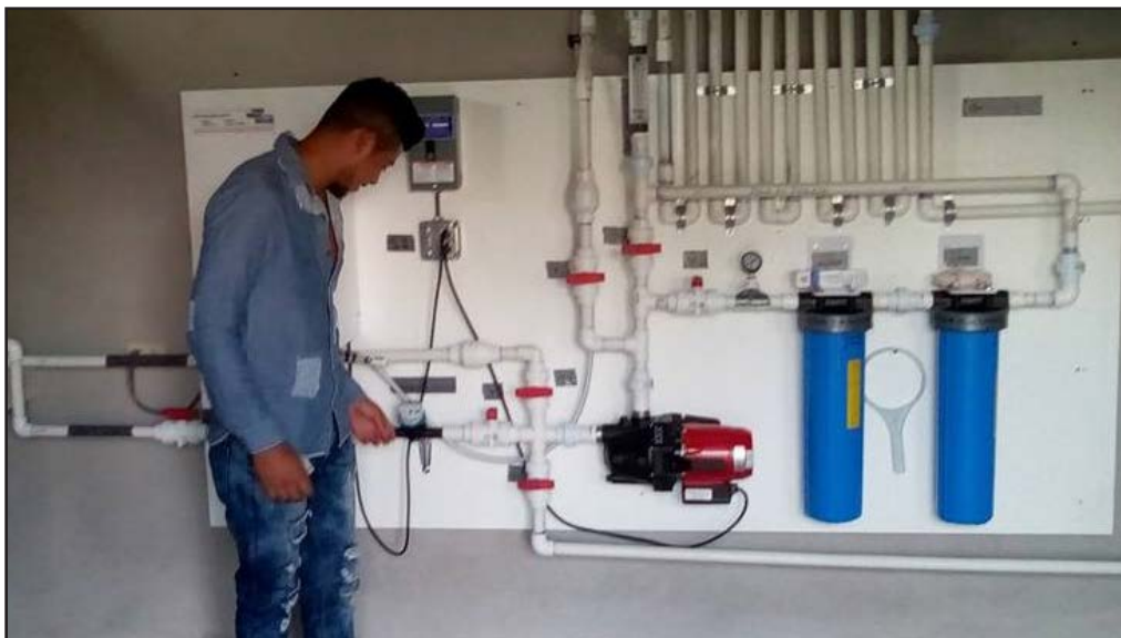
System operator Wilmer Torres Guerra checks the gauge on the LWW system installed by his community of La Pita, Honduras, and Broad Street UMC. The system uses filtration and ozone disinfection to make the water safe for consumption.
