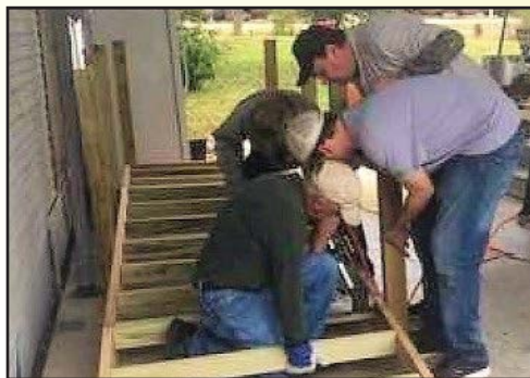
Men of First UMC build components for four handicap ramps completed in 2016.
