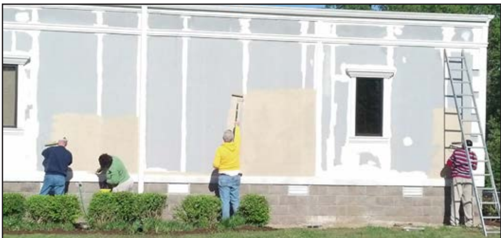
Men of Northside UMC paint the building housing "Hands Up," a program for at-risk children.
