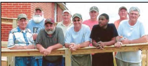
Men of Main Street UMC stand on a new 65-foot ramp they built for a Clio UMC.
