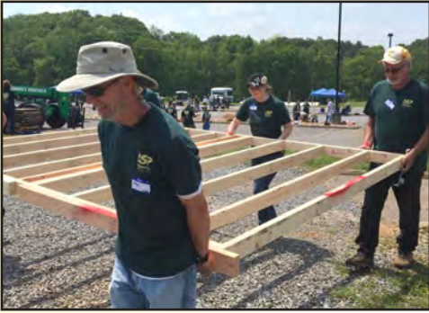
Volunteers carry the framing of a wall for a new house in Gatlinburg.
