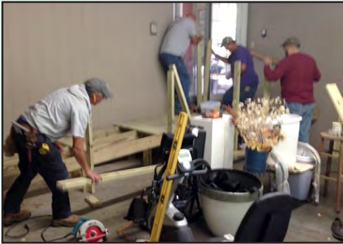
Men of Tabernacle UMC install a ramp for a church member. Photo by Jodie Plyler.
