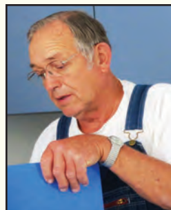
Larry Bolick installs a plexiglass screen between a baby-changing area and a sink in the Child Development Center at Mt. Bethel UMC in Hickory, N.C. He has spent countless hours making sure the center passes local and state codes.
