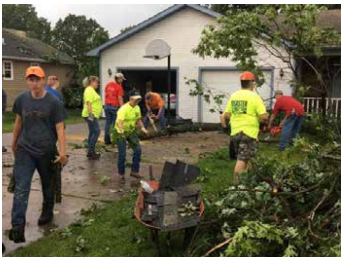
Some 30 members of Christ's Community UMC in Joplin saw up tree limbs and place tarps on roofs of Carl Junction homes damaged by a May tornado.
