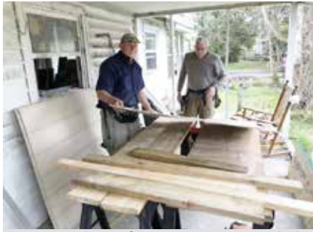
Two members of Cape Hatteras UMC help repair a flooded home in Ocracoke Island.
