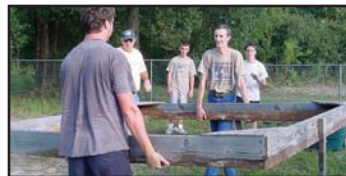
Kenneth Harrison and Ted Kimmel, Eagle Scouts from Troop 91, remove old playground material prior to building a new one. The new playground was an Eagle project led by John Watson Jr.
